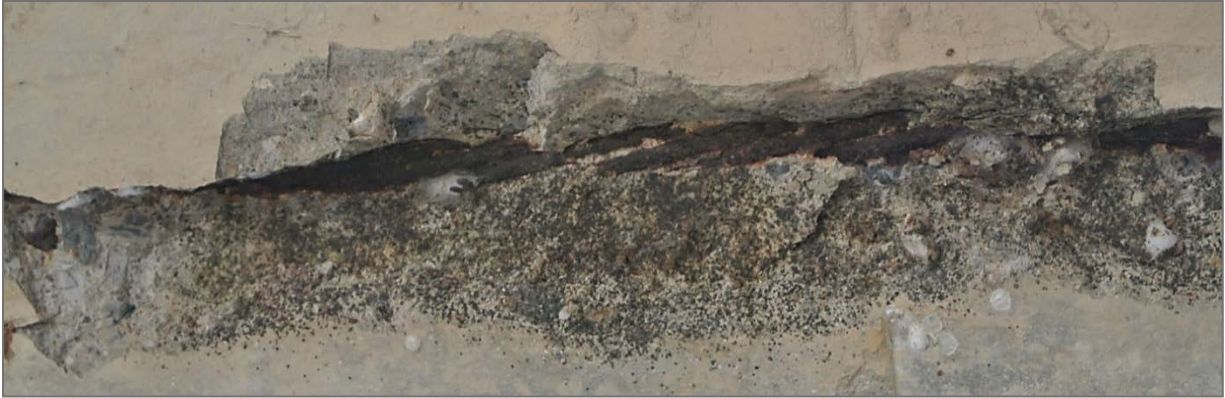
Figure 8.9 Spall on Girder C with exposed prestressing strand just south of midspan
