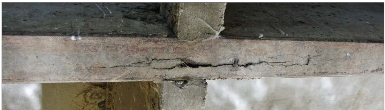
Figure 8.6 Longitudinal crack on Girder B at midspan
