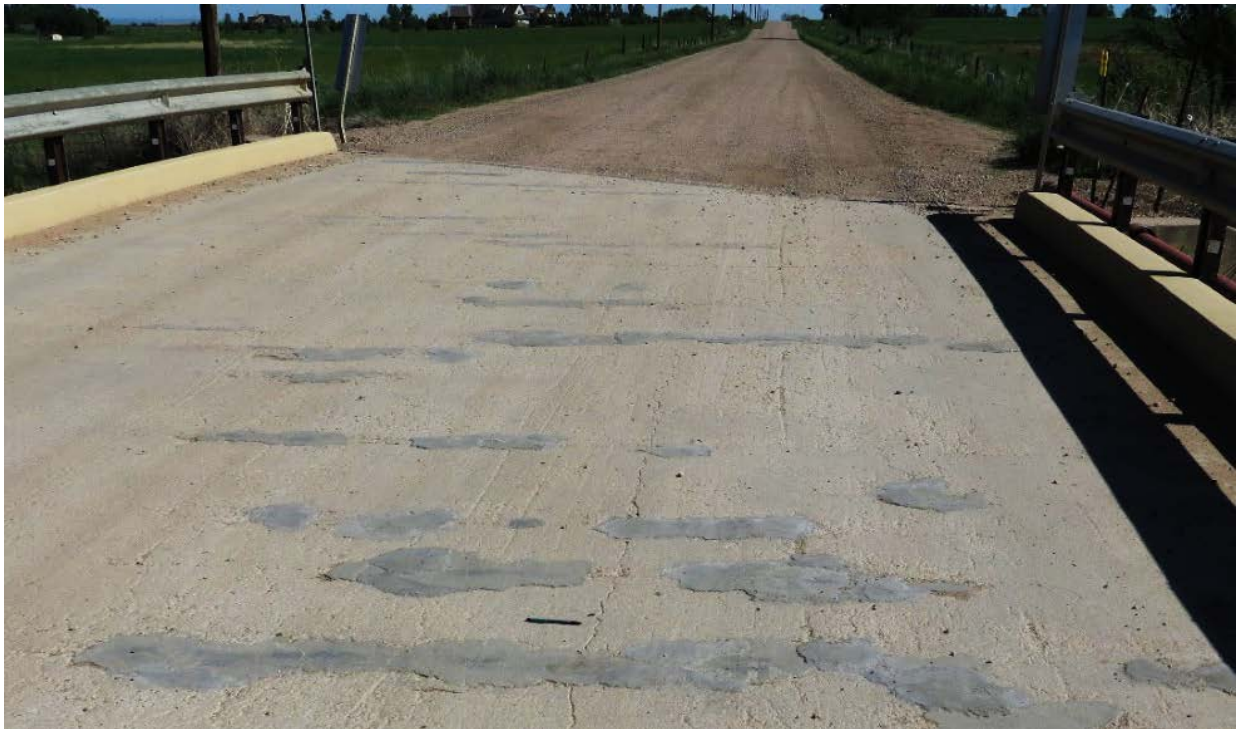
Figure 8.4 RC deck with longitudinal and transverse cracking
