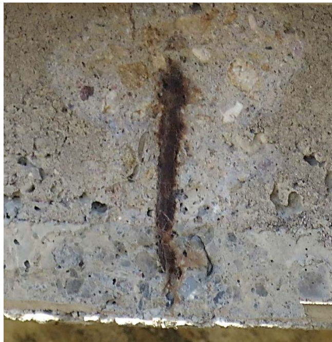
Figure 8.10 Spalling with exposed shear reinforcement on Girder C just south of midspan.
