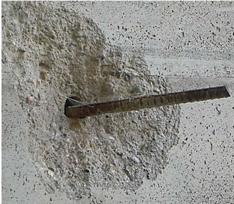
Figure 8.11 Large spalled region on Abutment 1
